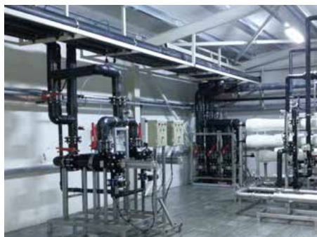
Two Bernoulli Filters remove large harmful particles from sea water before the ultrafiltration membrane system in a desalination plant.
