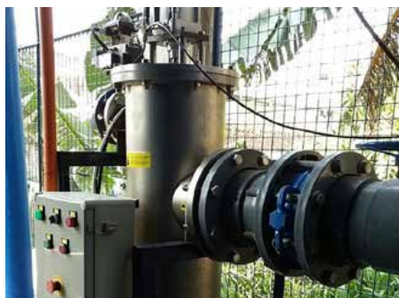
A Bernoulli Filter is working in a waste water treatment system as a pre-filter removing large particles.
