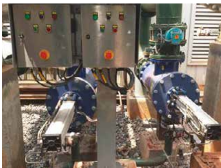
Two Bernoulli Filters are installed before plate heat exchangers to reduce clogging and fouling in a power plant.
