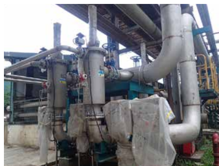
Four Bernoulli Filters are working parallelly to purify raw river water which is supplied to the paper mill as process water.
